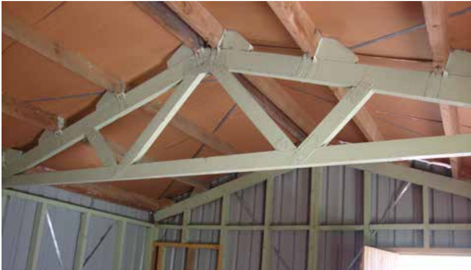
This house survived unscathed from TC Winston, when nearly all else around it was destroyed. Note strapping on every joint, diagonal bracing on the wall and roof panels and metal plates on the truss timbers. (Source Habitat for Humanity)
